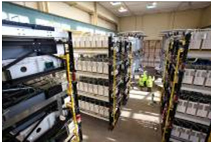
25 MW demonstrator with back-to-back converters commissioned
